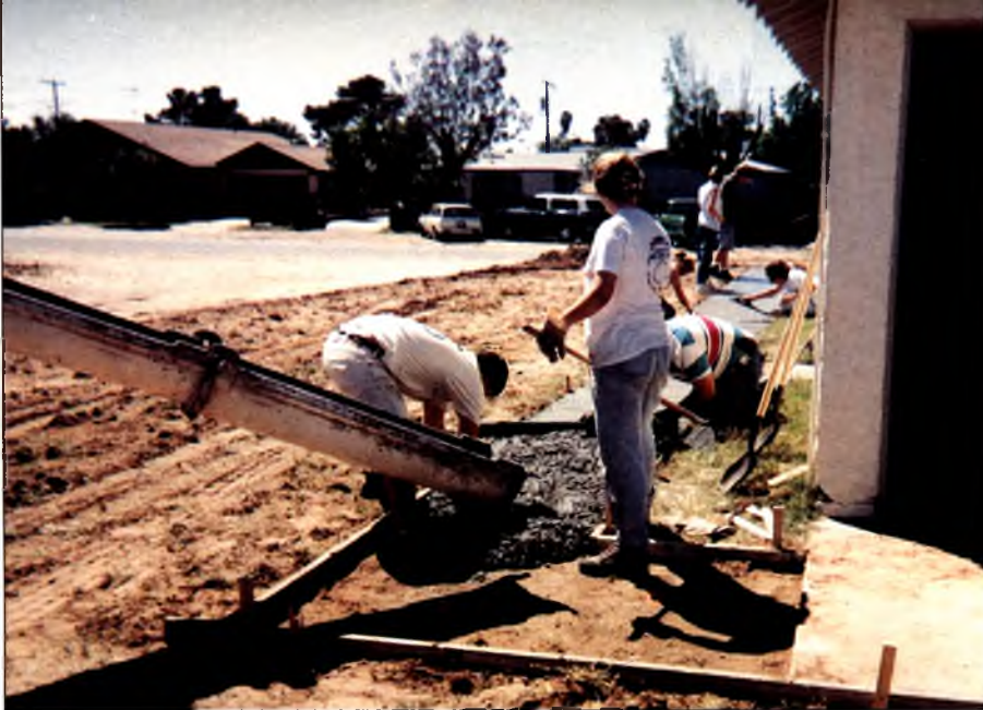
When the concrete pours, you don't even have time to look up and smile for the photographer. Project YES involved PLNC students in a variety of construction tasks working with Native Americans.
