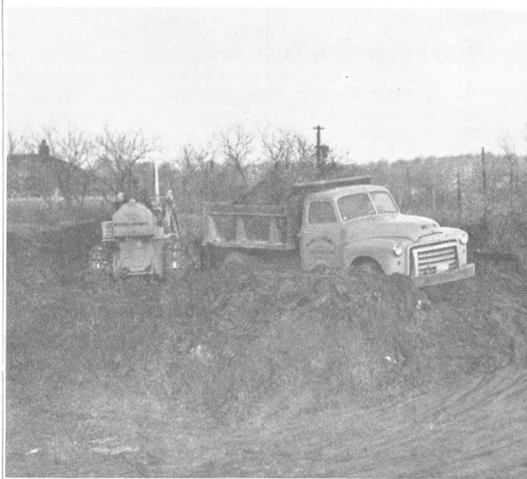
Excavation and landscaping for Fine Arts Building on campus quadrangle. Other excavating is being done for commercial site on four-lane boulevard, and for industrial site near Tennessee Central Railroad.
